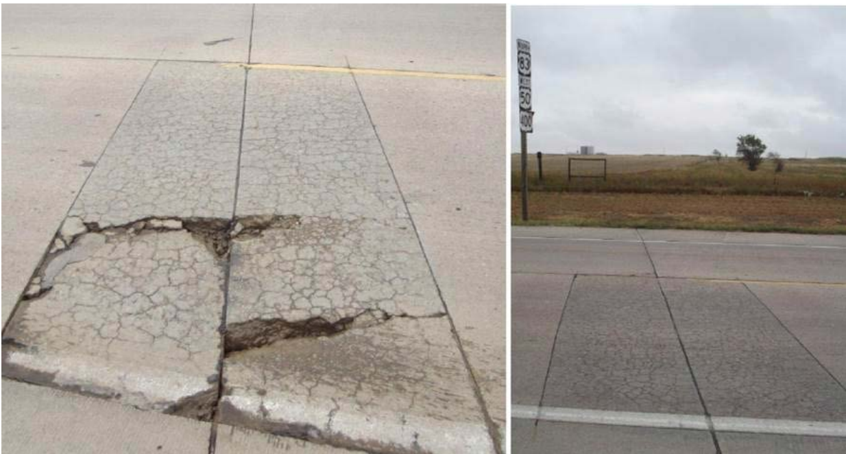
Figure 1-4: Prematurely Deteriorated Slabs in Garden City, Kansas (photo courtesy of Rodney Montney, KDOT)
