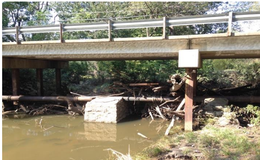
Figure 17: Madison Street bridge and pipe displaying a large amount of debris collection. PT-2 was located on the other side of the debris pile from where the photographer is standing.
