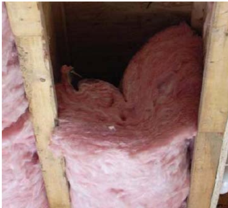
Figure 6-1 Improperly installed roof insulation. Photo courtesy of SIPA.
