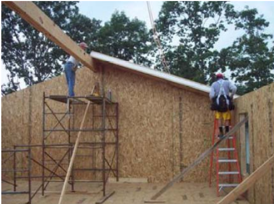
Figure 4-4 Roof panels are installed with drying in the structure. Photo courtesy of SIPA.
