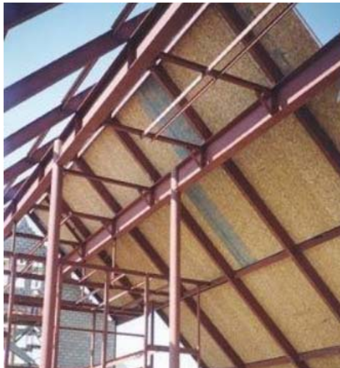
Figure 2-3 Building with a steel frame and SIP roofing and wall panels. Photo courtesy of SIPA.
