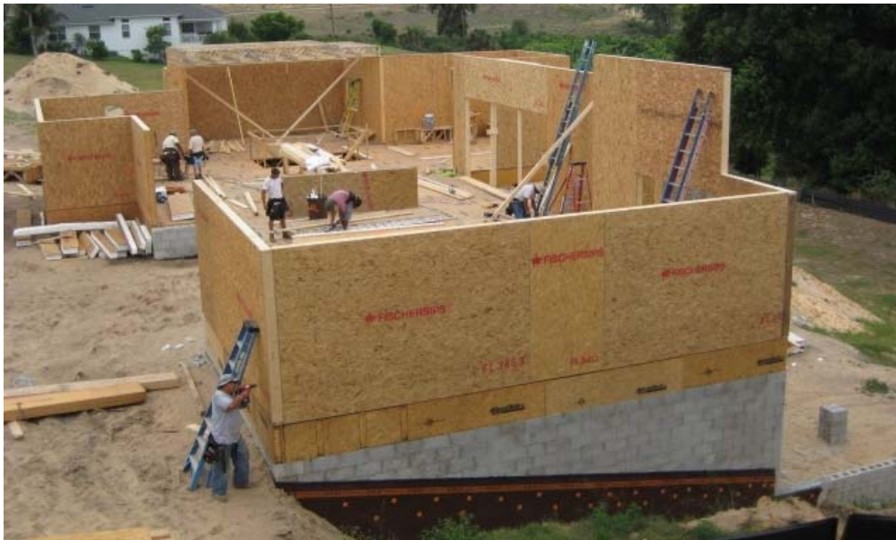
Figure 6-6 Construction site of a new SIP house. Photo courtesy of Fischer SIPs.
