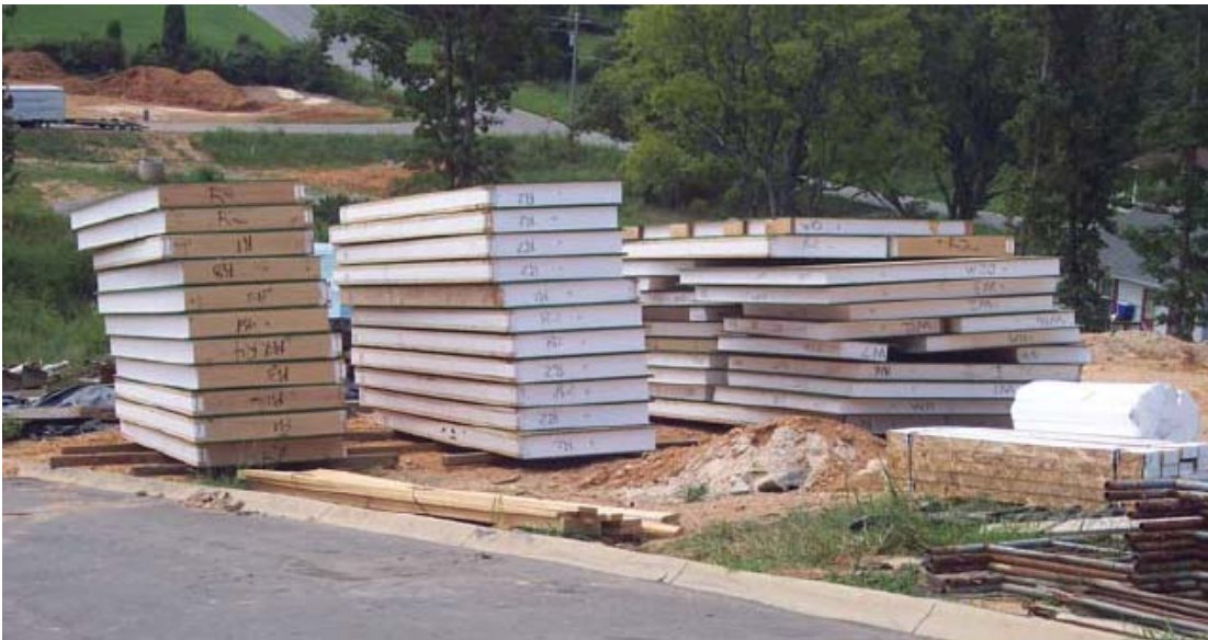
Figure 4-1 Panels stockpiled on site ready to be installed. Photo courtesy of SIPA.
