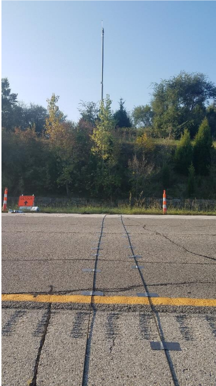
Figure 32 Road Tube Configuration Below Data Collection Tower
