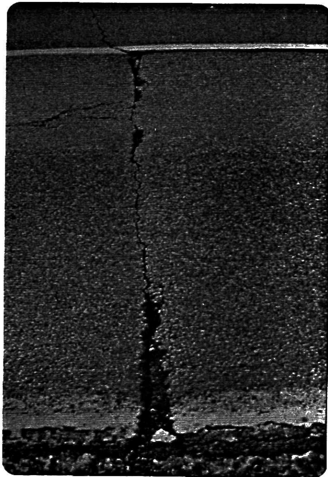
Fig.12. HIGH SEVERITY TRANSVERSE CRACK (From U S Dept. of Transportation and Federal Highway Administration, 1984.)
