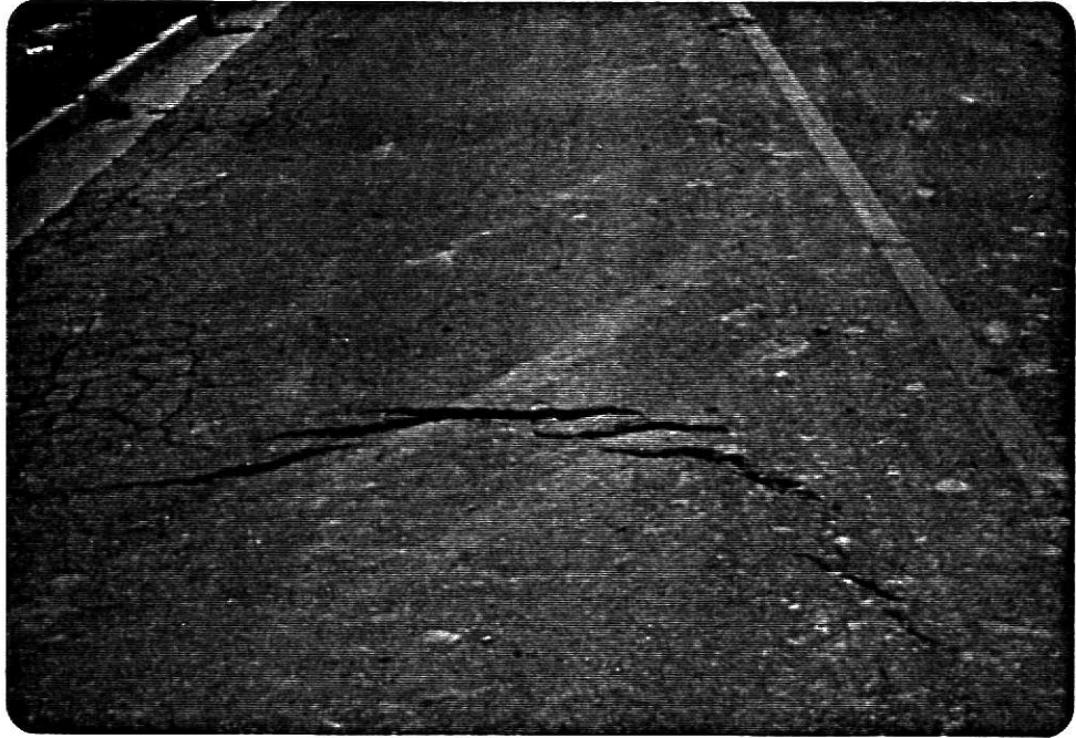
Fig. 13. SLIPPAGE CRACK. (From The Asphalt Institute, 1983.)
