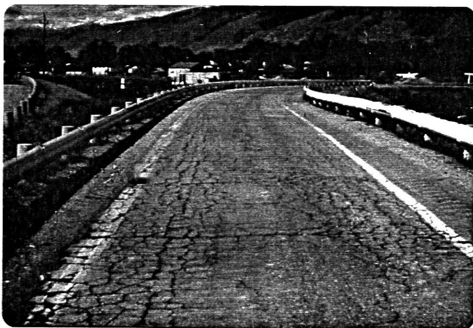
Fig. 7. HIGH SEVERITY FATIGUE CRACKING. (From U S Dept. of Transportation and Federal Highway Administration, 1984.)
