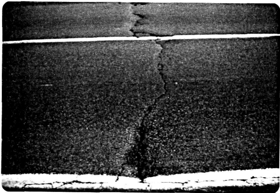
Fig. 11. MEDIUM SEVERITY TRANSVERSE CRACK. (From The Asphalt Institute, 1983.)
