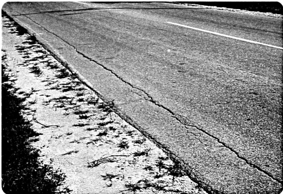
Fig. 9. EDGE CRACKING. (From The Asphalt Institute, 1983.)
