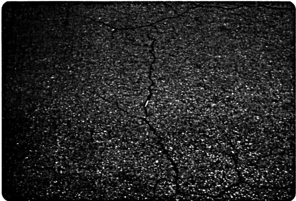
Fig. 14. REFLECTION CRACK. (From U S Dept. of Transportation and Federal Highway Administration, 1984.)
