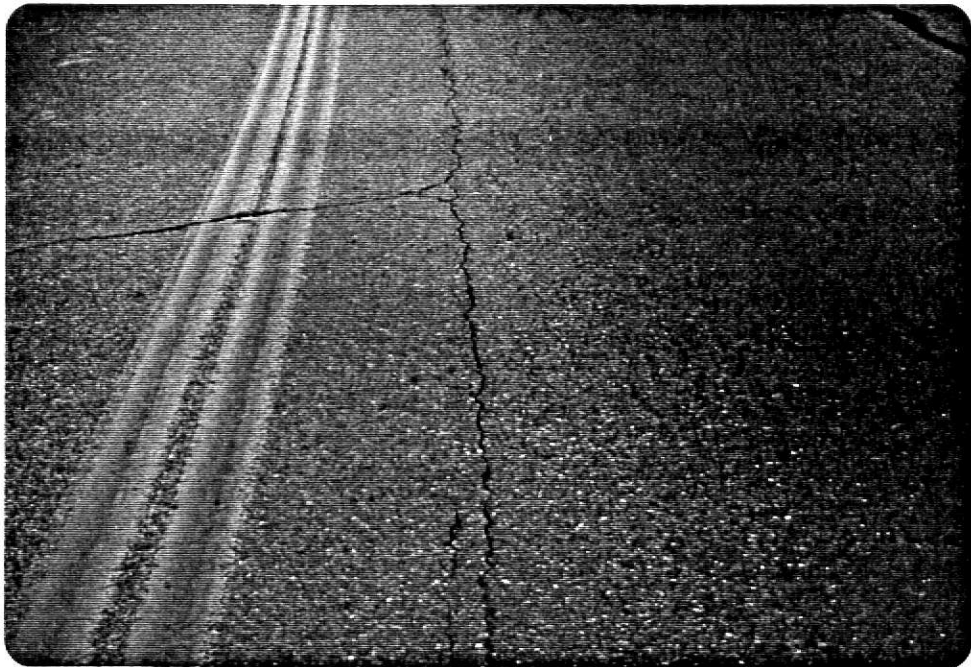
Fig. 8. LONGITUDNAL AND TRANSVERSE CRACK. (From U S Dept. of Transportation and Federal Highway Administration 1984.)
