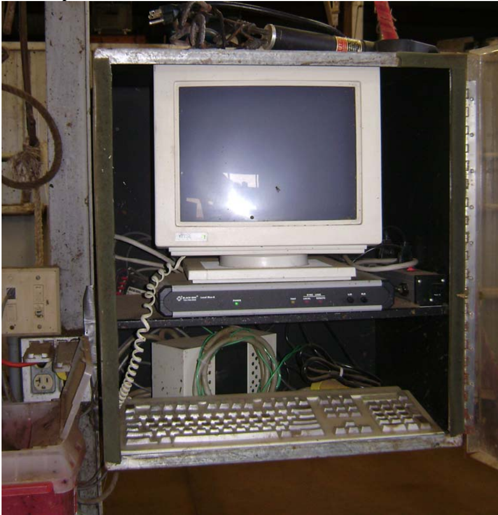
Figure 5.19 Knight Feed Yard, Picture of computer and black box, noted in Figure 5.16, cause of potential interference
