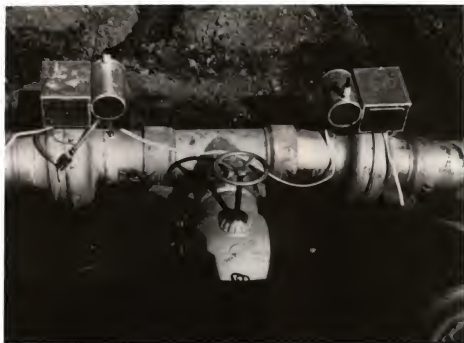
Figure 3. Flow Control Valves Mounted on a Riser.
