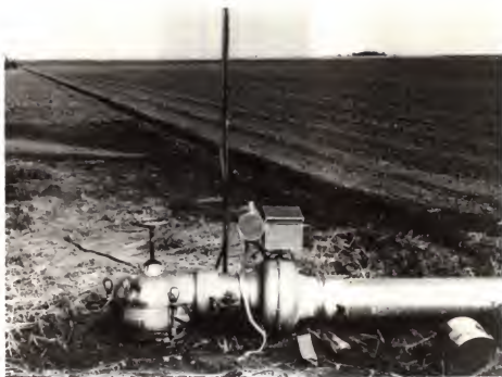
Figure 5. Safety Valve in Field.
