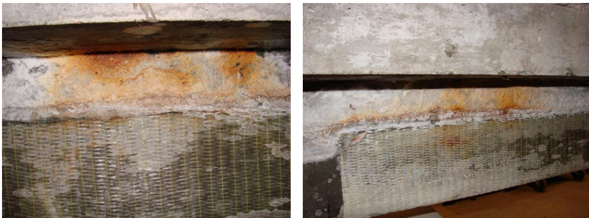
Figure 4-14: Some Red Stains at Beam T3 After Submerging in Deicing Salt Water.
