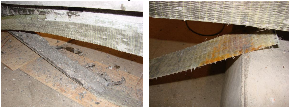
Figure 4-18: Cover Delamination Failure Followed by GFRP Debonding in T3.
