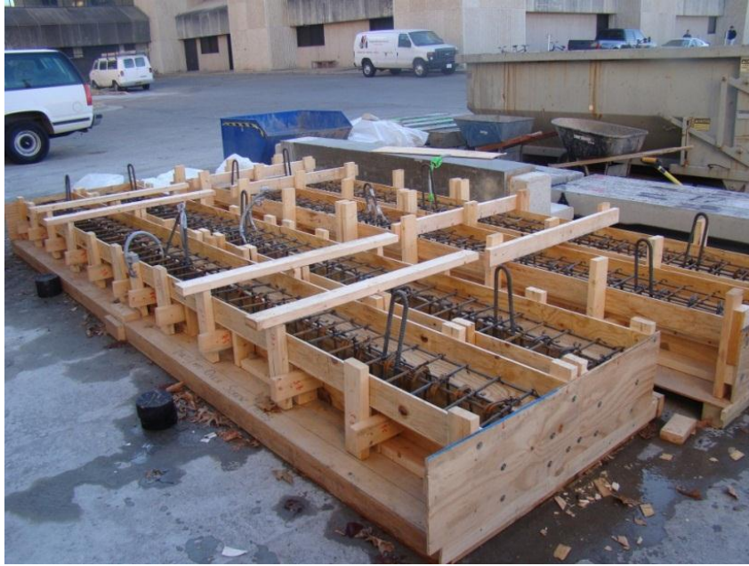
Figure 3-12: Top View of the Formwork with Reinforcement Cages In-Place for T-Specimen Casting.
