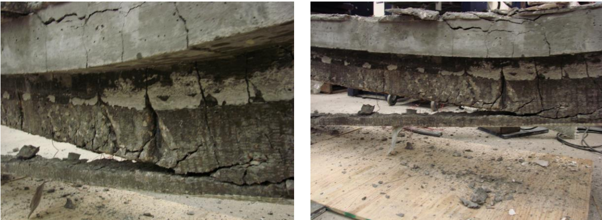
Figure 4-22: Failure of Beam T3
