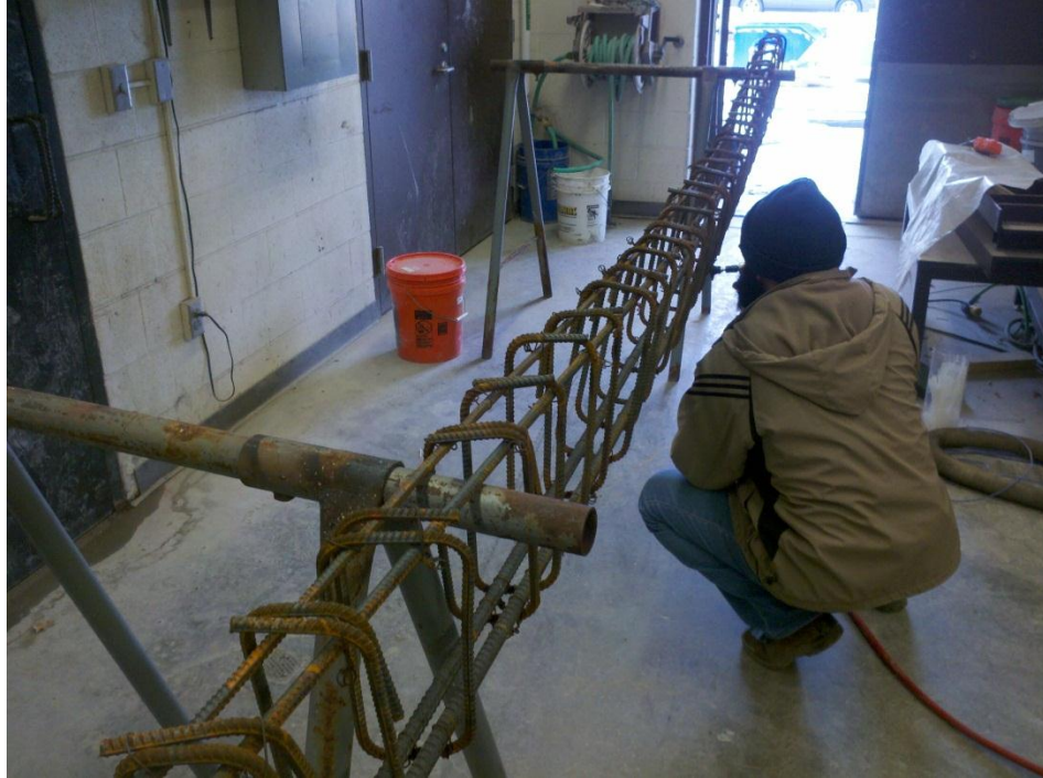
Figure 3-13: The Finished Rebar Cage Used for the Rectangular Part of The T Shaped Beams.
