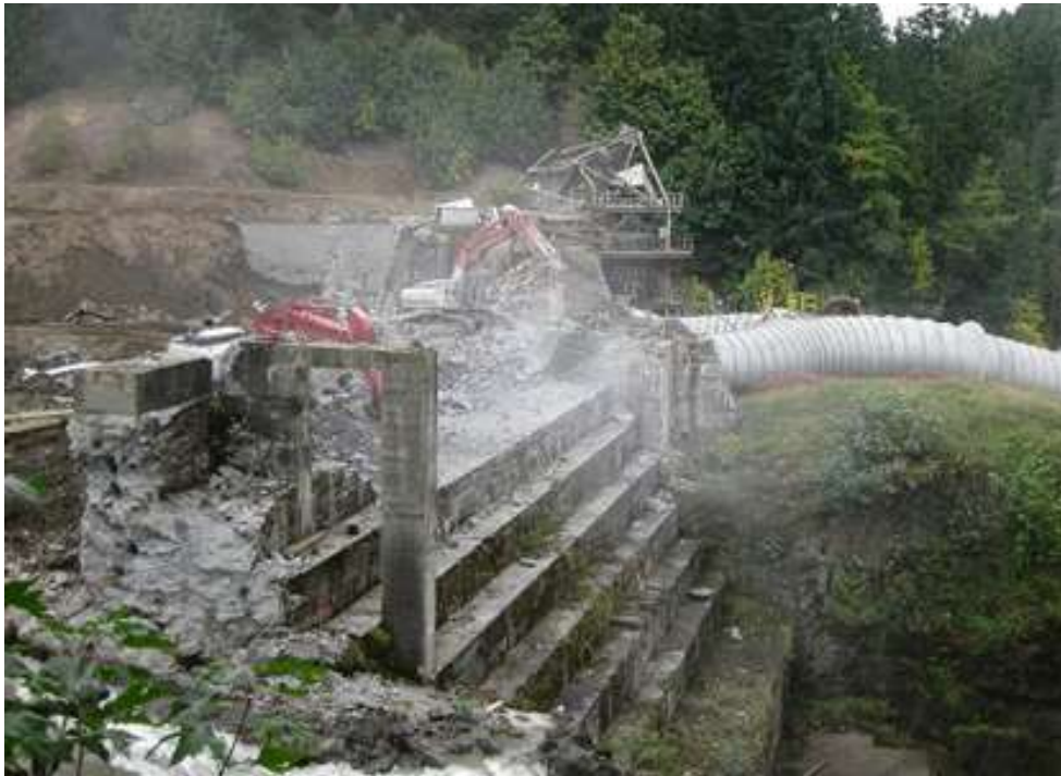
Figure 3.7. Demolition begins October 17 on the Elwha Dam using excavators. Here the machines are slowly removing pieces of the gravity section of the dam “recognizable by its stair-step appearance” (Olympic National Park Dam Removal Blog Archives 2011).
