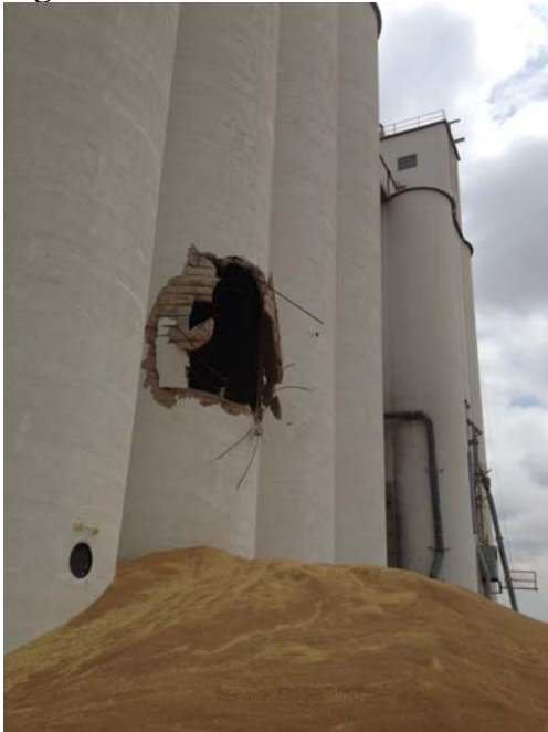
Figure 1.2: Wolf Elevator Bin Failure
