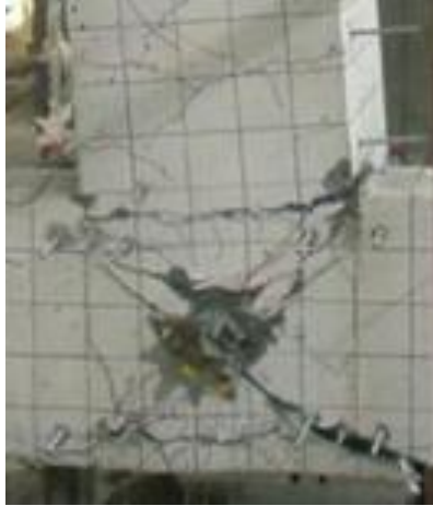
Figure 5.3-5: Damage due to Shear Loading. Reprinted from ‘Innovative Techniques for Seismic Retrofit of RC Joints’ by I. Bedirhanoglu, A. Ilki, N. Kumbasar, 2015.
