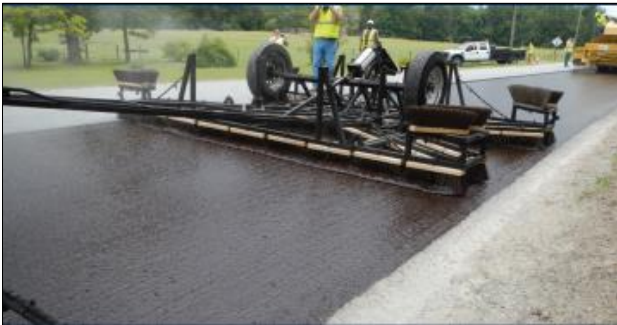
Figure 6-4 Application of scrub seal with scrub seal brooms placed at different angles (National Center for Asphalt Technology a )
