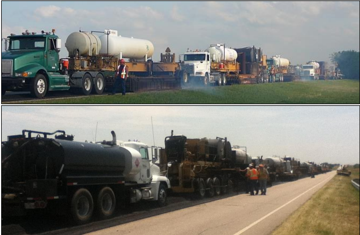
Figure 1-3 HIR train (preheating and heating and recycling units)
