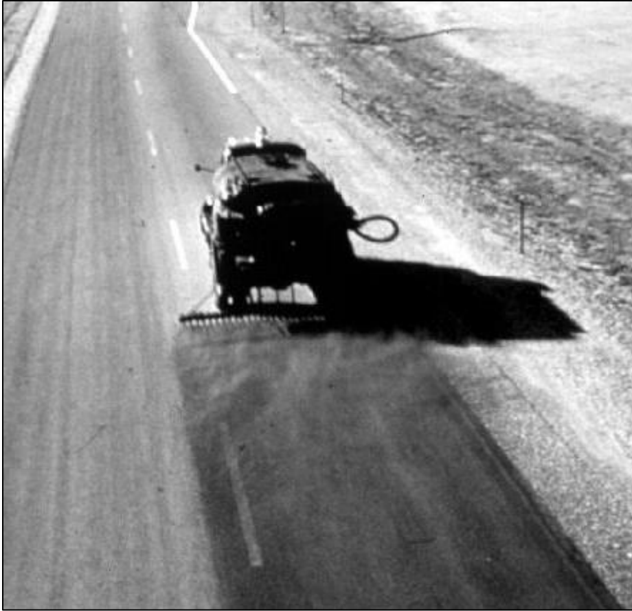
Figure 6-2 Application of fog seal on the asphalt concrete pavement (U.S. Forest Services)
