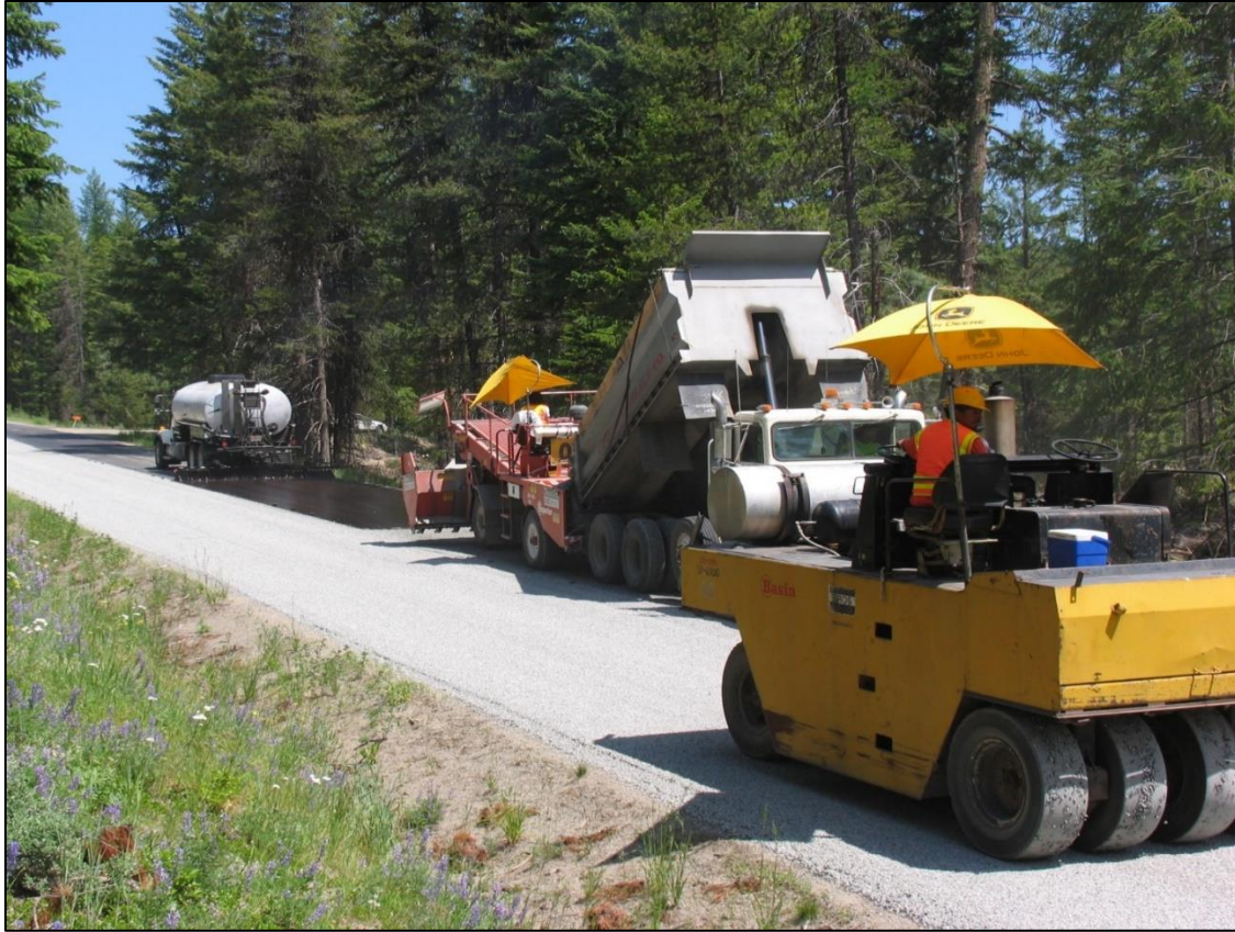
Figure 6-5 Application of chip seal: asphalt emulsion applied first, followed by chip spreader (driving backwards) and roller (pavement interactive)
