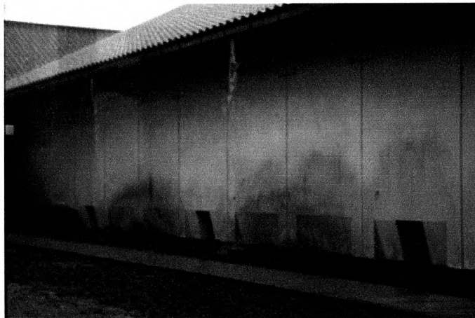
Fig 3.7: The rain running through the holes of gutter creating water fall.
