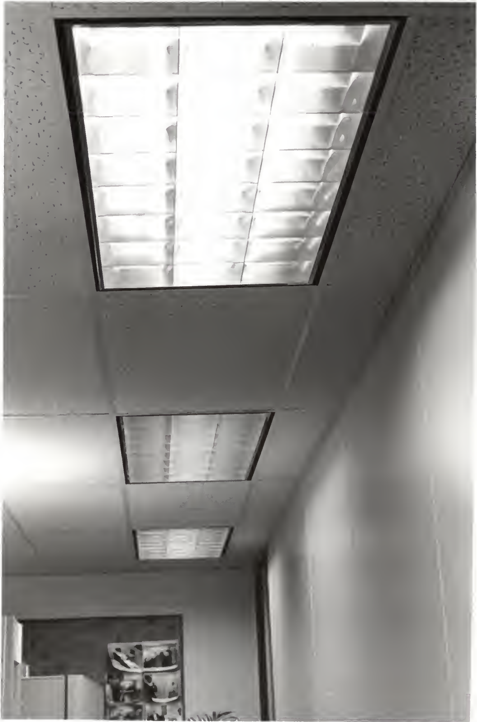
Figure 1. Louvered ceiling lights.
