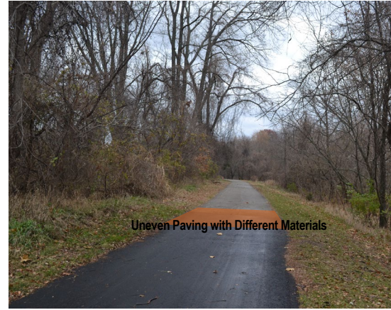
Figure 4-34 | Patchwork of Pavement (Patterson, 2014)
