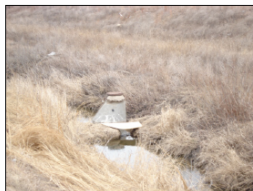
Image 4: Exposed manhole cone shows depth of erosion since its installation (date currently unknown).
