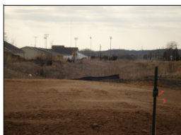
Image 5: First major bend in channel. Based on evidence of grading, a new house is proposed for this site with limited buffer zone between the channel and structure.
