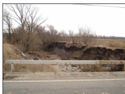
Image 6: Channel erosion that has occurred beyond the boundaries of upstream residential development.
