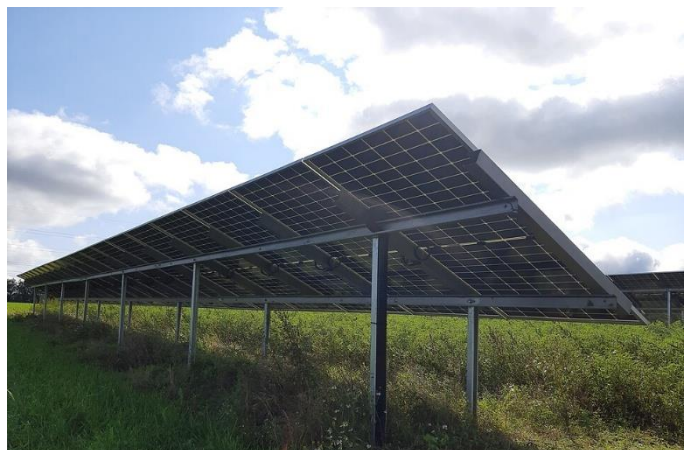
Figure 10 - Victoria, M. (2023, August 26). Fixed mounting structure in a photovoltaic array [Photograph]. Wikimedia Commons. https://commons.wikimedia.org/wiki/File:Fixed_mounting_structure_in_a_photovoltaic_array.jpg
