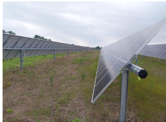
Figure 11 - Uniaxial-tilt tracking array outside of Lawrence, KS
