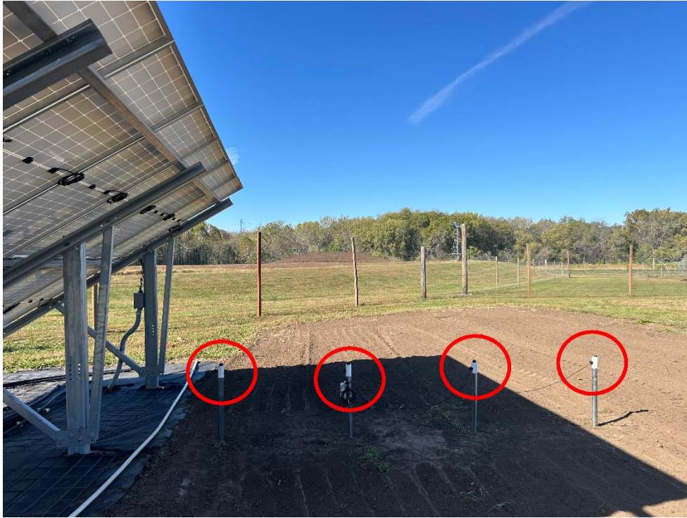
Figure 30 - Sensors (circled in red markup) placed behind panel array at LT site.
