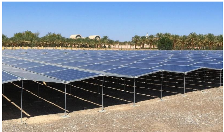
Figure 17 - "East-West Array". Image by Jurchen Technology, accessed October 20, 2025, from https://www.jurchen-technology.com/peg-design/ . Used under Fair Use rights. No modifications made.
