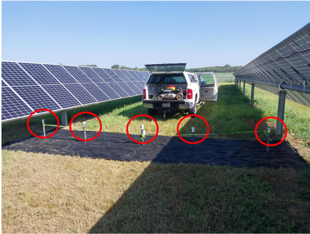
Figure 33 - PAR sensors (circled in red markup) between uniaxial-tracking arrays at UT site in Douglas County, KS
