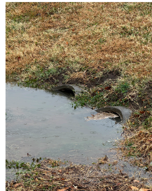
Fig 5.9 Current drainage pipes are filled by off-site sediment, leaves, and debris causing clogging during large rain events (Freelove 2024).
