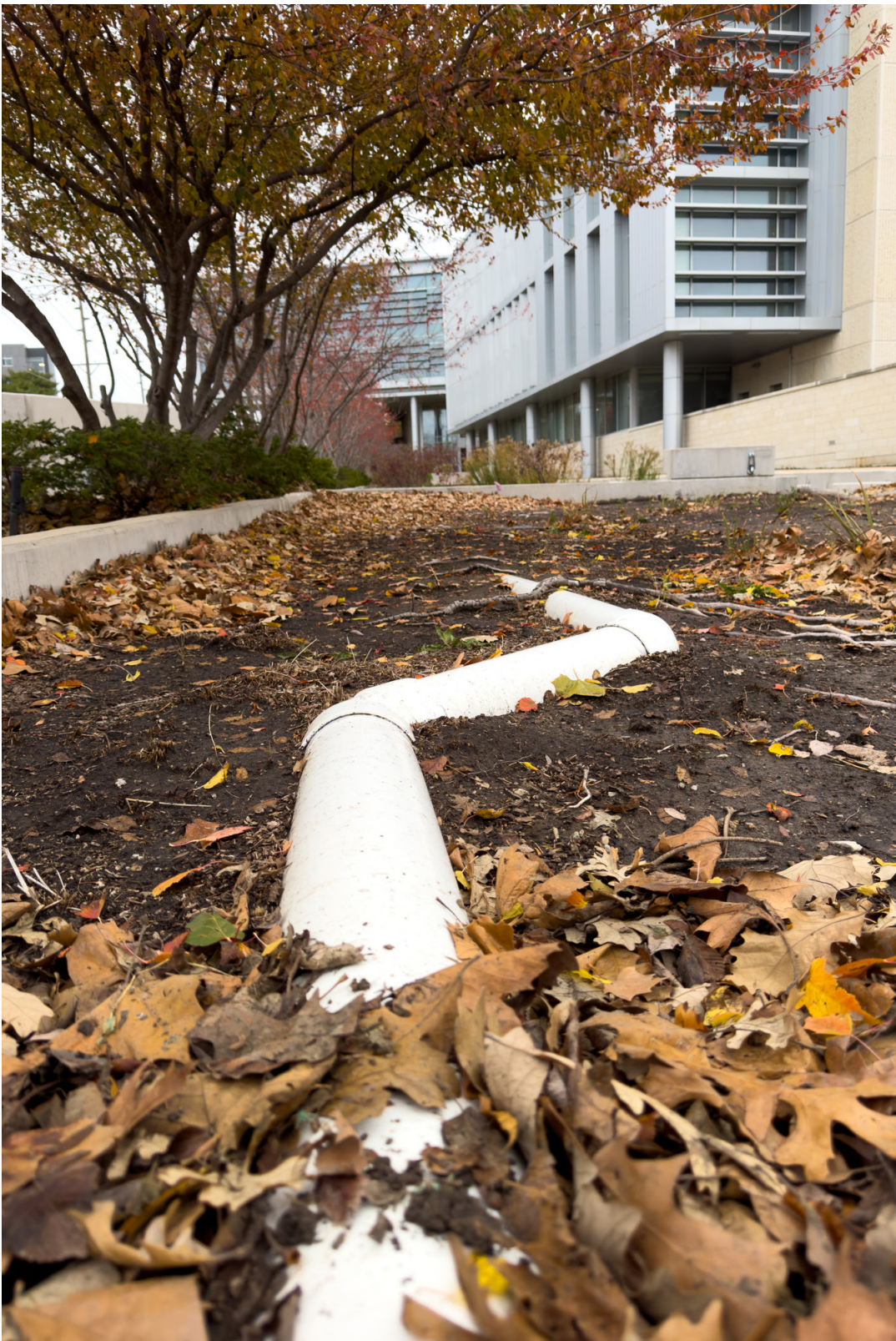
Fig 6.3 Exposed piping in lowest Engineering Bio-Retention Cell at Kansas State (Freelove 2024).
