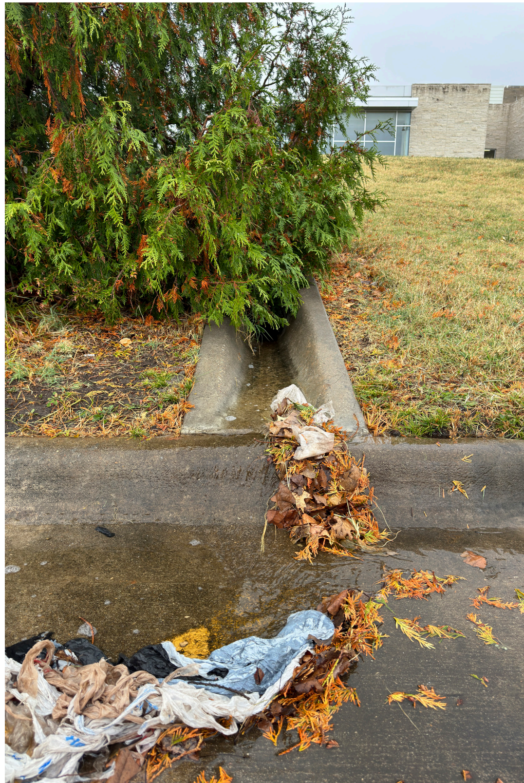
Fig 5.7 Edwards Hall currently has some areas where stormwater expels onto the parking lot, then flows into storm drains without any stoppage (Freelove 2024).
