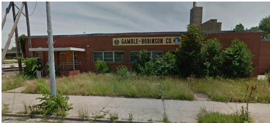
Figure 4.7.4 - Deteriorating Building Facade (Johnson, 2019)
