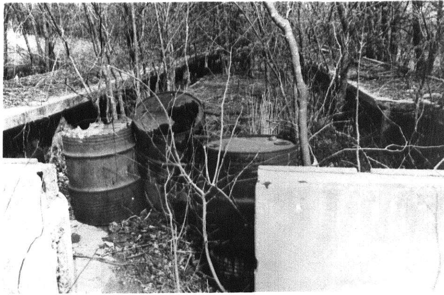
Figure 24. The Greenhouse Foundation is Heavily Overgrown with Tree Saplings.
