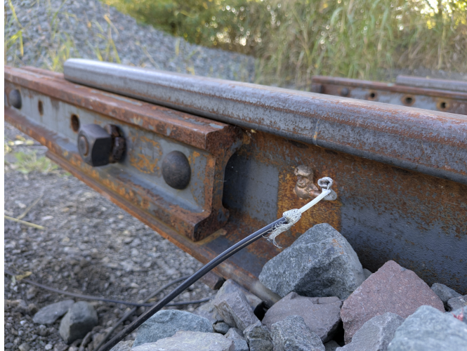
Figure 2.2: Photo of Cable Connection Point on Track
