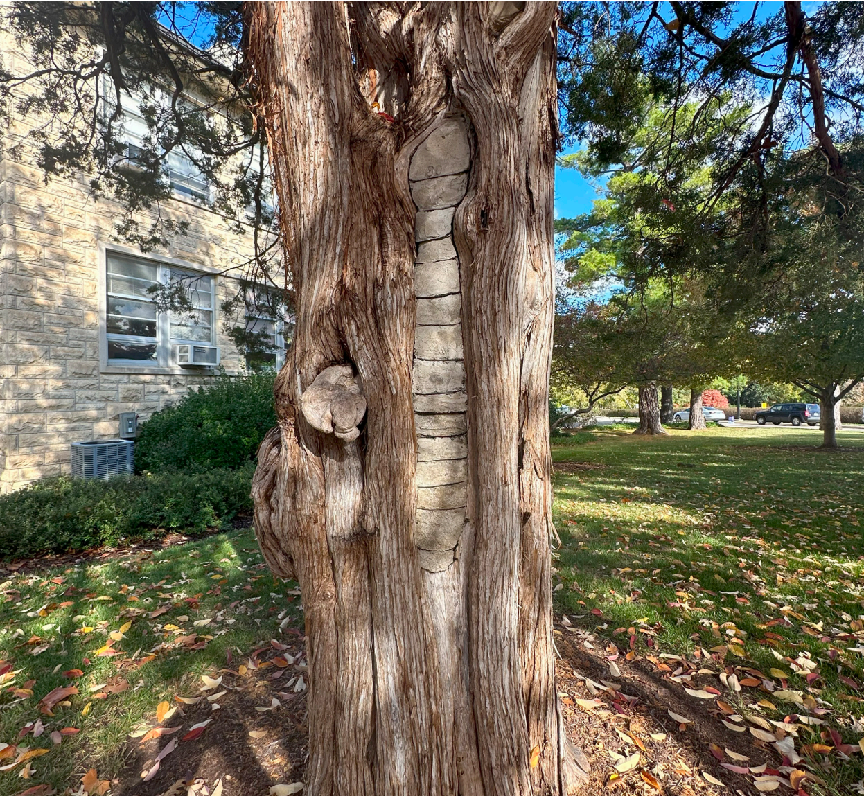
Figure 2.17 Shows a cavity in an Eastern Red Cedar tree filled with concrete. While this was once thought to stop decay and support the tree, experts now advise against filling cavities unless necessary. These concerted efforts were made to preserve and protect the K-State campus trees (by author).
