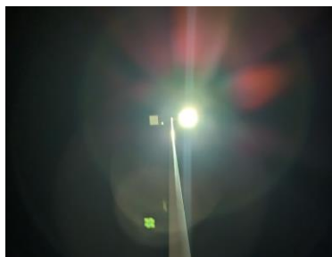
Figure 37 - Pole mounted fixture
