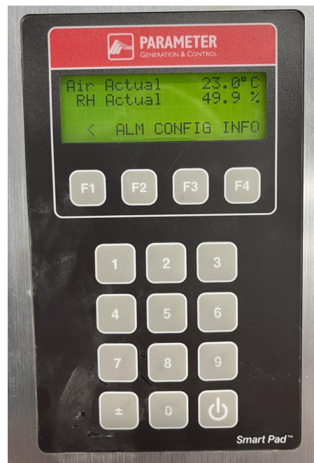
Figure 12. Testing room environment control panel
