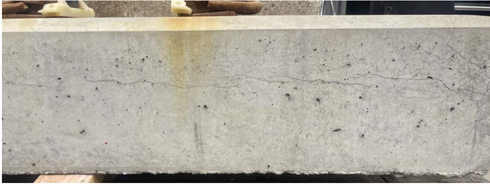
Figure 21: Post-2003 Cracking at 90 Freeze-Thaw Cycles
