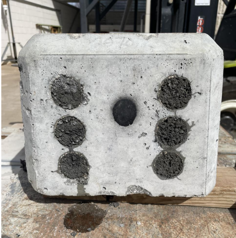
Figure 29: Water Seepage of PT Tie
