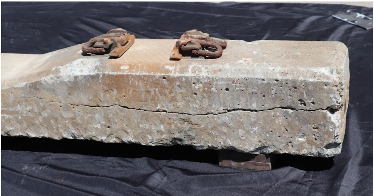
Figure 2: Pre-existing Damage of Pre-2003 Tie
