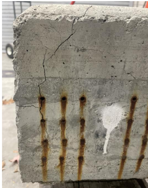
Figure 22: Post-2003 End Slip
