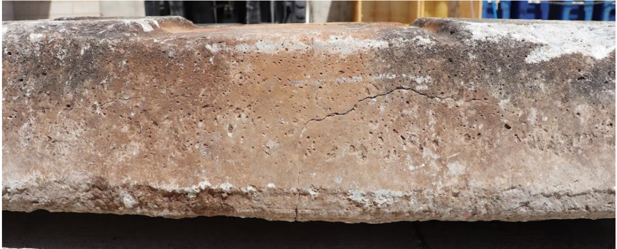
Figure 1: Pre-existing Damage of RCCC Tie
