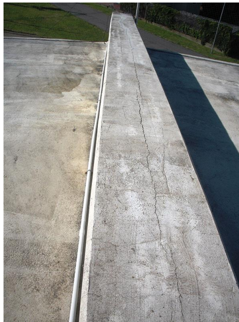
Figure 8. Concrete Degradation Characterized by Alkali–Silica Reaction Cracking (Barnes & Zamora, 2015)
