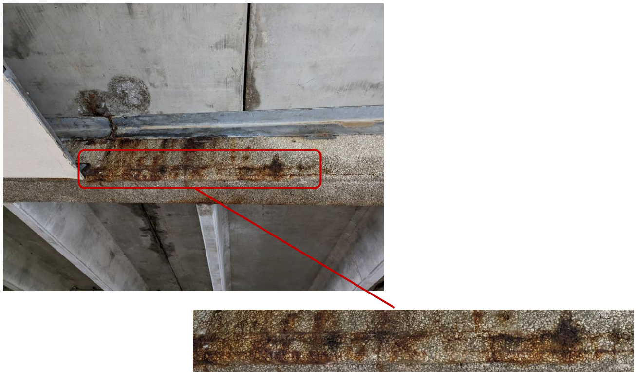
Figure 10. Concrete Degradation Associated with Chloride Ingress, by ASM Engineering Consultants (Est. 2007)
