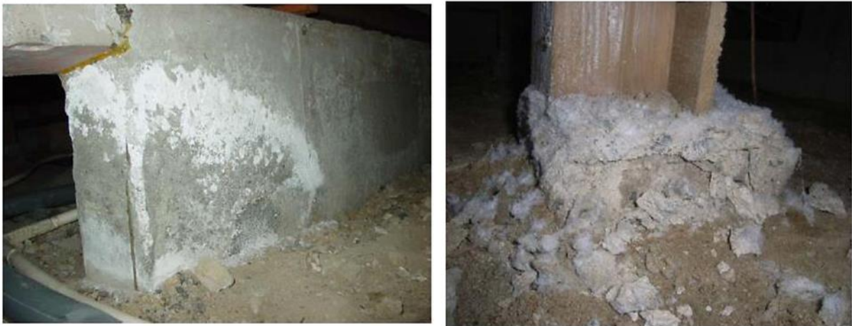
Figure 9. Concrete Degradation Caused by Sulfate Attack and Salt Crystallization (Skillsite, 2023)
