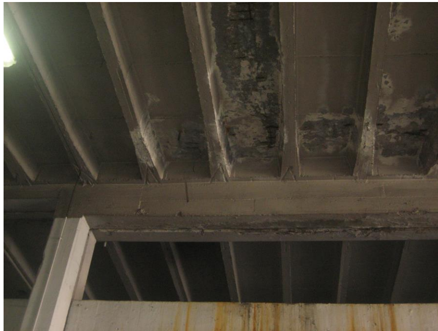
Figure 4. Carbonation-Induced Degradation of Exposed Concrete Surfaces, by ASM Engineering Consultants (Est. 2007)
