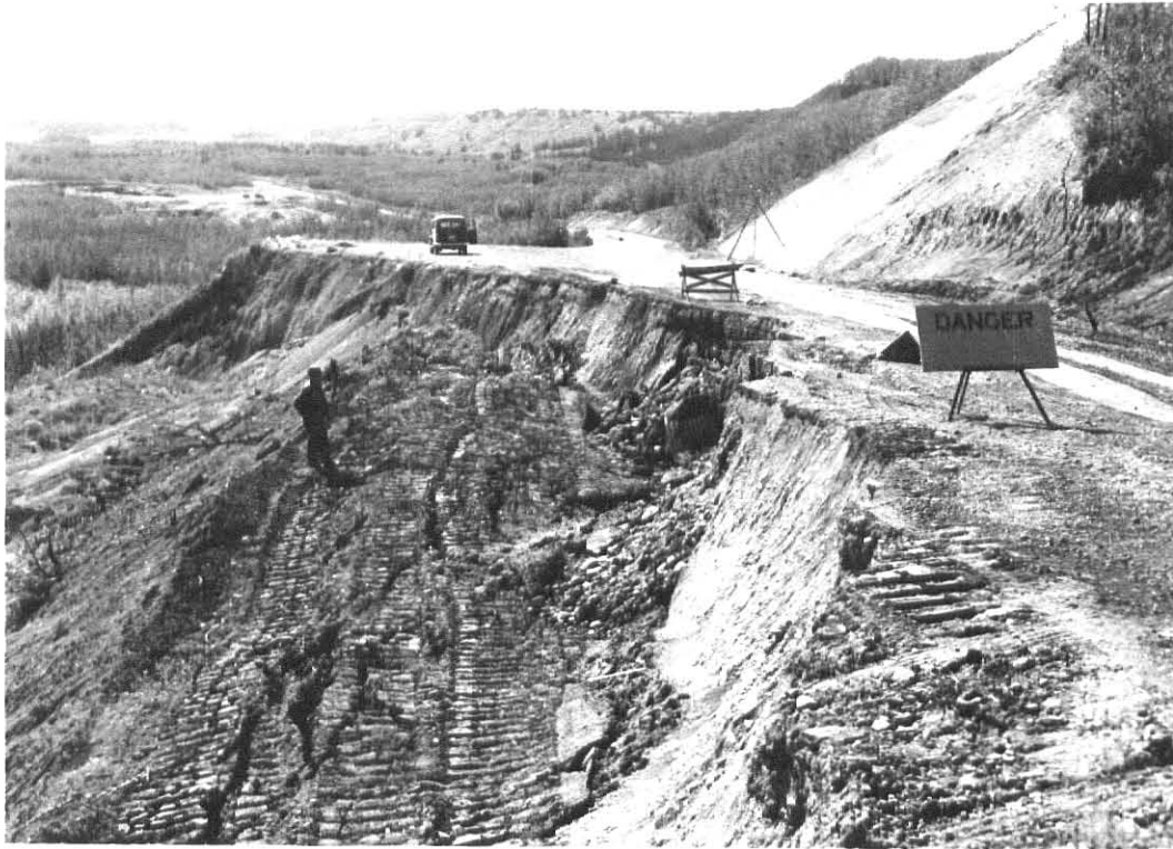
Fig. 6. Slump block of fine grained highway fill material at Simpson Hill, on the Richardson Highway. Centerline of road formerly lay over exposed part of sheared culvert. Note bulldozer tracks on slump block surface, which are a continuation of those at road level on right side of photograph. Photo courtesy Department of the Interior.
