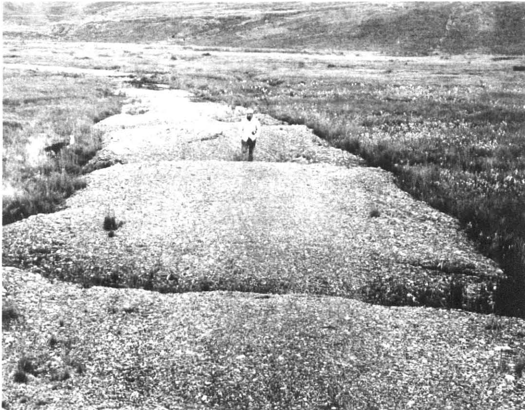
Fig. 7. Gravel road near Umiat showing severe differential subsidence caused by thawing of ice-wedge polygons in permafrost. Photo courtesy Department of the Interior.
