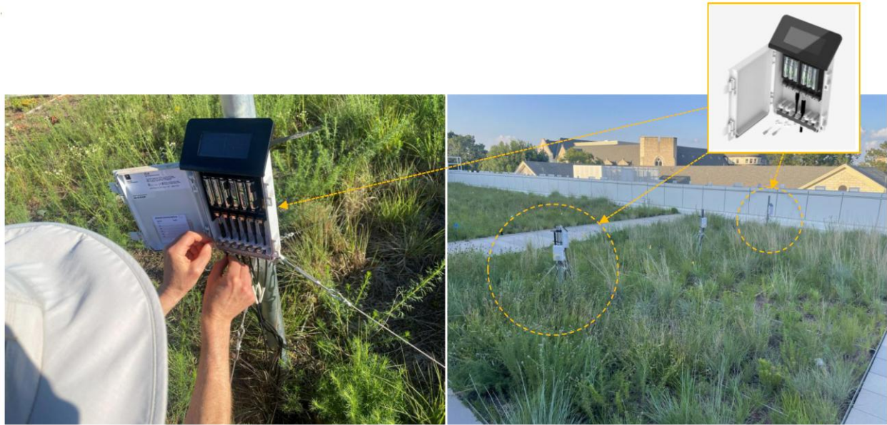
Figure 3.9: Connecting sensors with data loggers.
