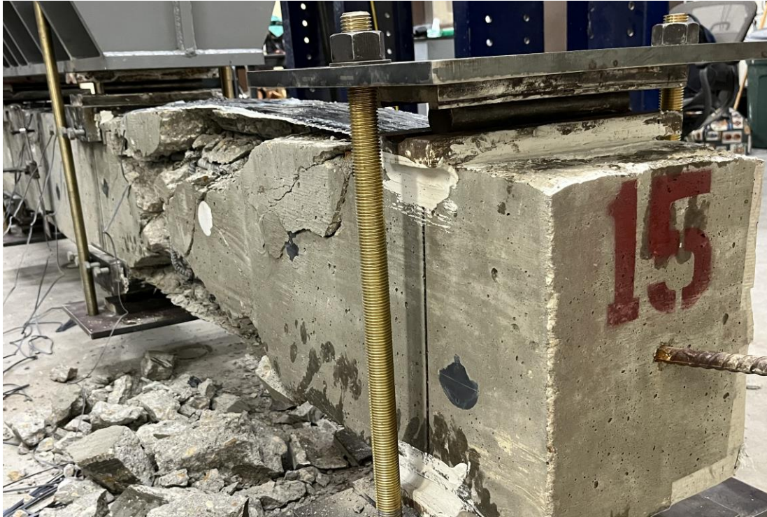
Figure 5.26. Failure Mode of beam No.15.
