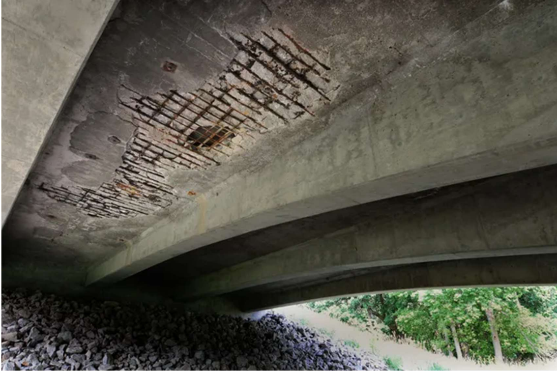
Figure 2.1: Underside view of a reinforced concrete bridge deck showing concrete spalling and exposed corroded reinforcement (Salina Journal, 2015)
