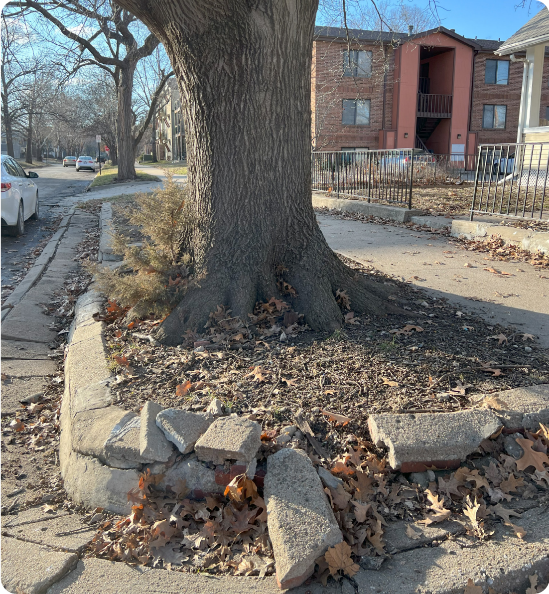
Figure 4.14 Constrained tree roots causing cracked and lifted curbs (Saunders 2024). Planting pits should be designed to be big enough so that tree roots do not interfere with the surrounding hardscape.
