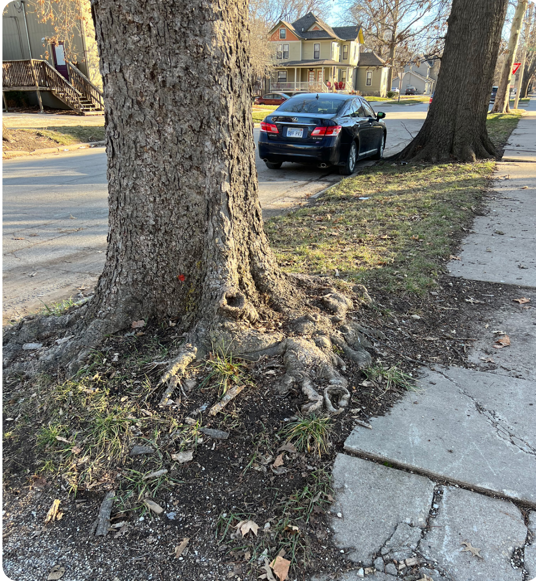
Figure 4.13 Constrained tree roots causing lifted and cracked sidewalks (Saunders 2024). If tree trunks and sidewalks are too close to each other, roots can severely damage the sidewalk, presenting tripping hazards.
