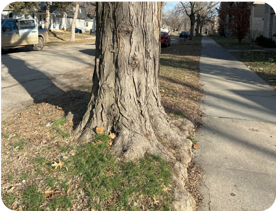
Figure 6.1 Tree roots interfering with sidewalk (Saunders 2024).
