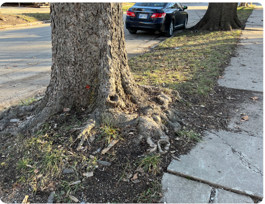
Figure 6.4 Tree roots lifting and cracking adjacent sidewalk (Saunders 2024).
