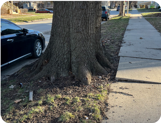
Figure 4.34 Damaged sidewalk (Saunders 2024).
