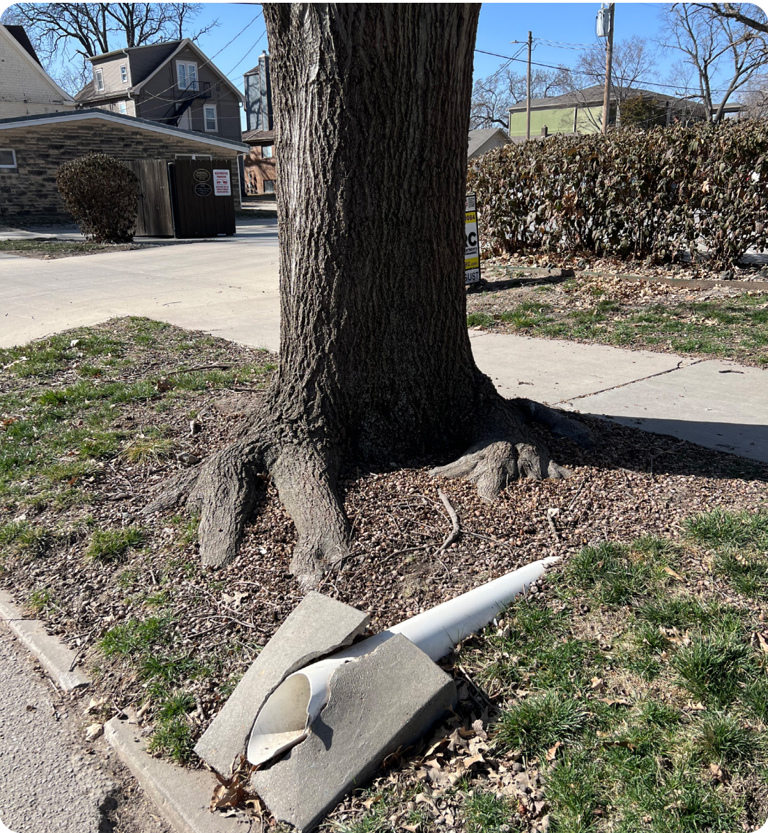
Figure 4.21 Large Street Tree Impacting Pipe (Saunders 2024). Utilities and trees should be considered with the same importance so they don't interfere with each other.
