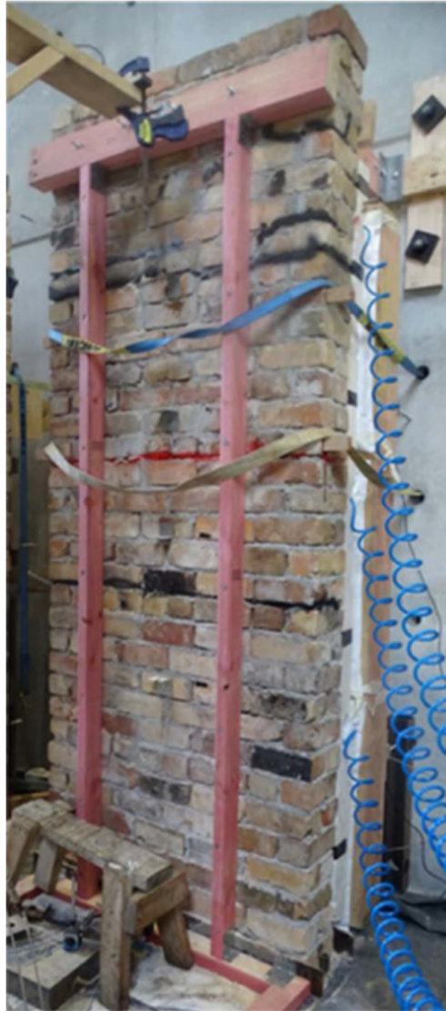
Figure 24: Timber Strongbacks on Wall
