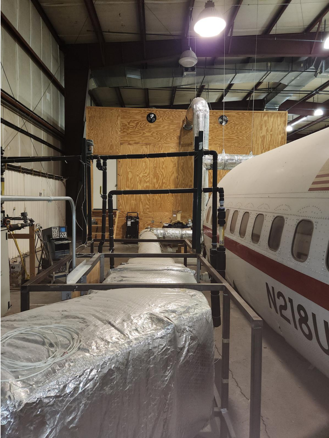
Figure 3.10: Exit Munters Ductwork
