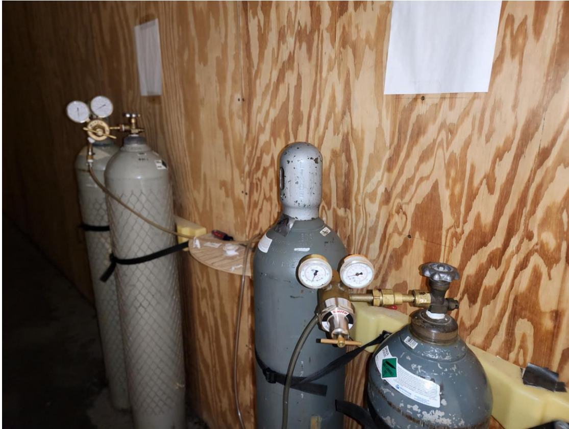
Figure 3.16: Gas Tanks with Regulators
