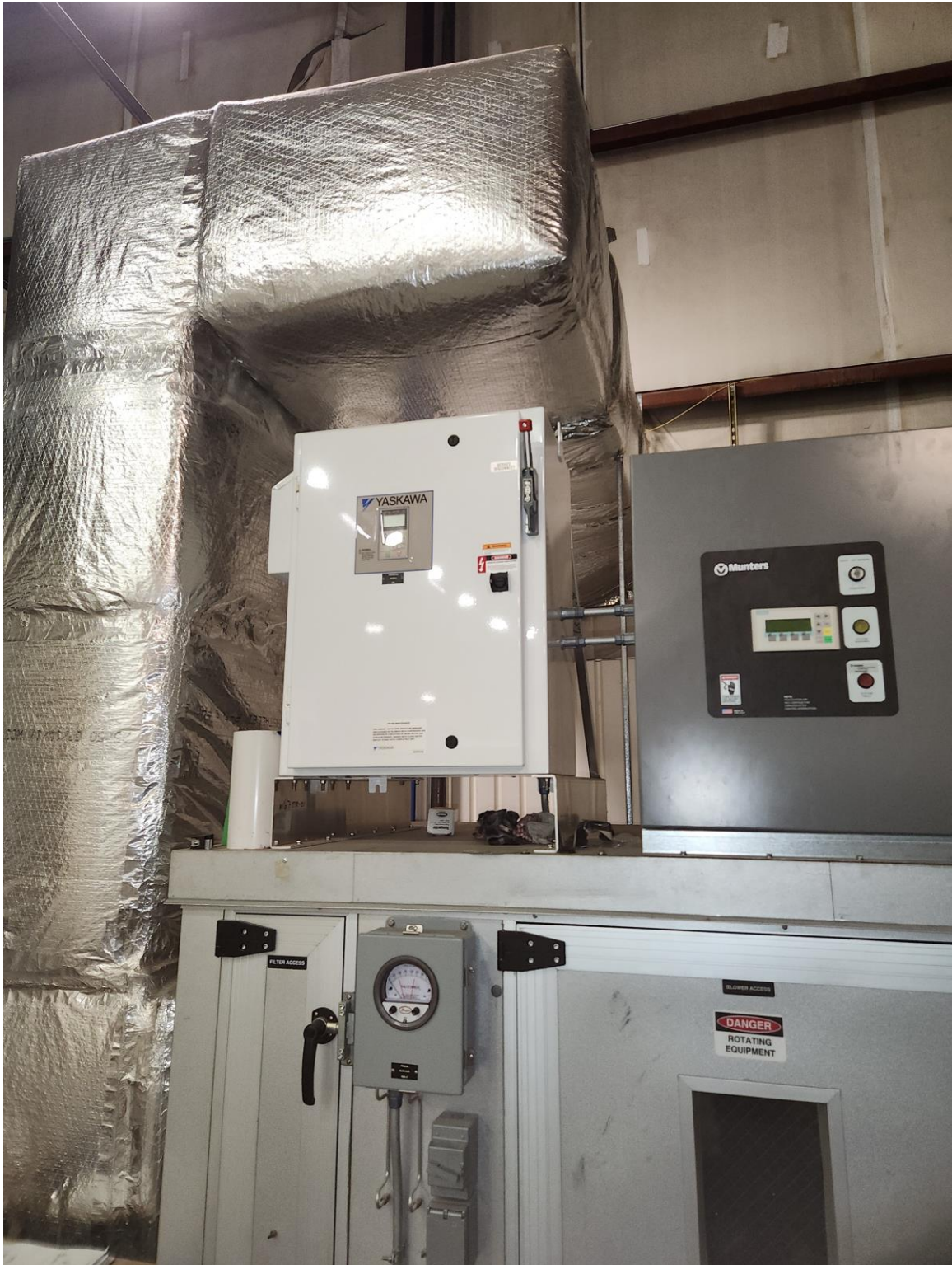
Figure 3.9: Entrance Munters Ductwork
