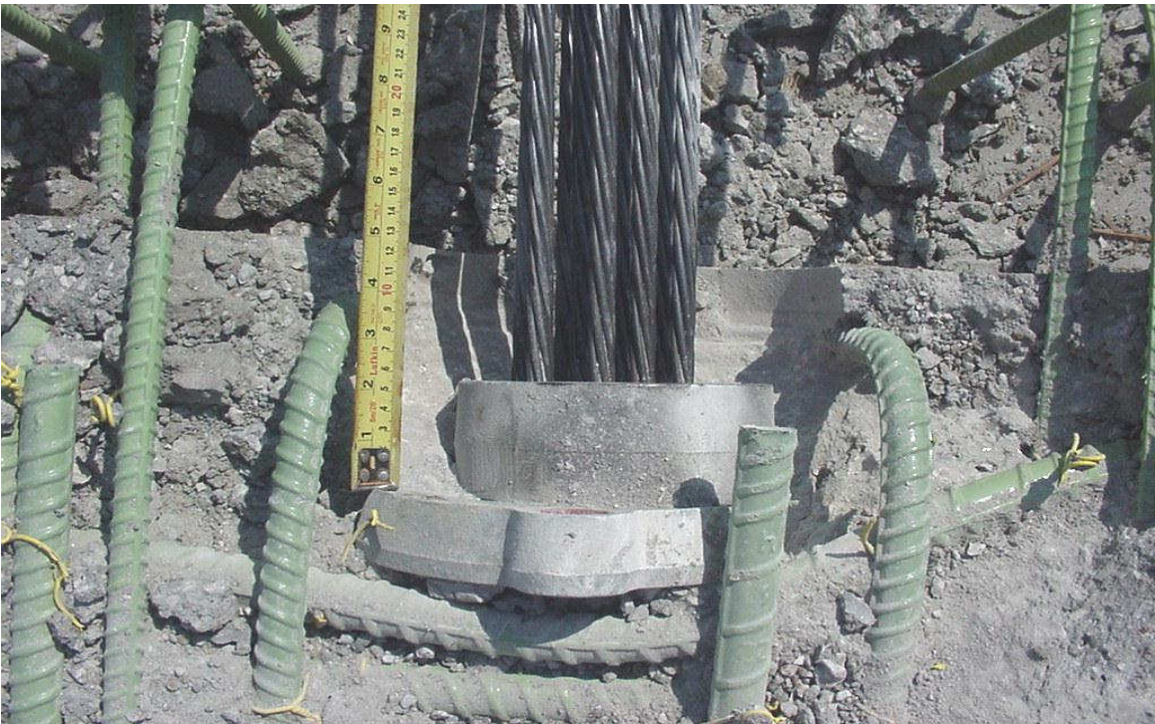
Figure 1.4: Close-Up View of Longitudinal Anchorage Point Failure (KDOT)
