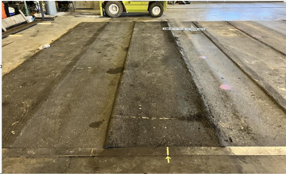
Figure 5.24 Rutting on Pavement Test Section Surface
