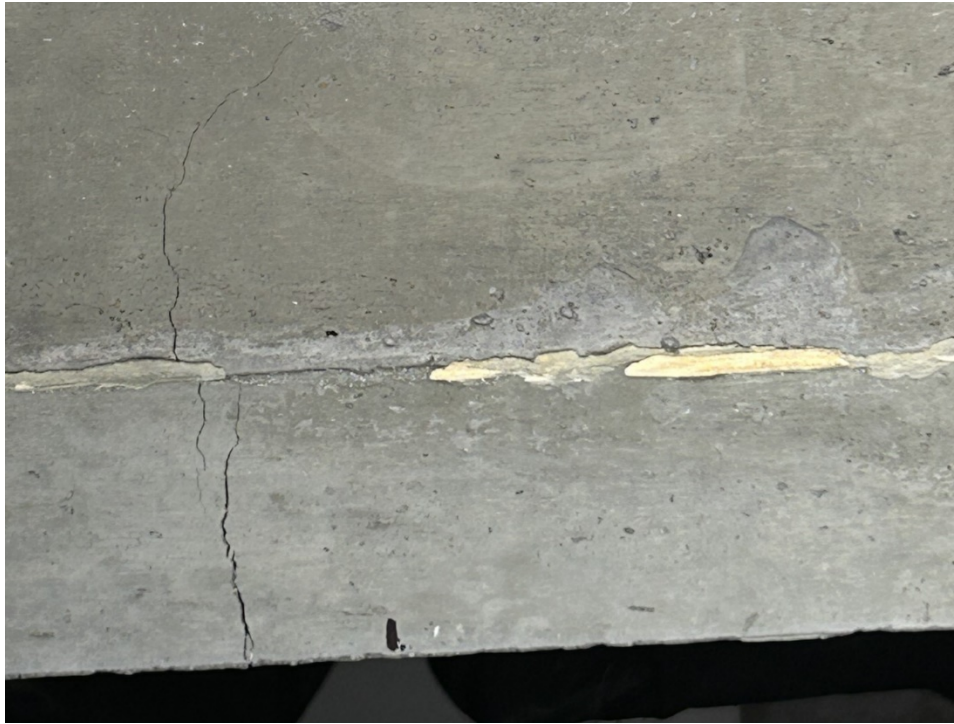
Figure 30: Crack at Plane of Panel and Topping
