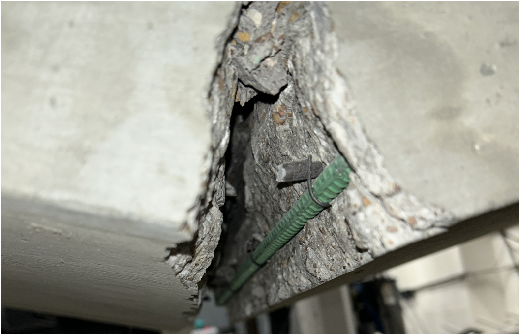
Figure 42: 6-ft T4-VAE Failure
