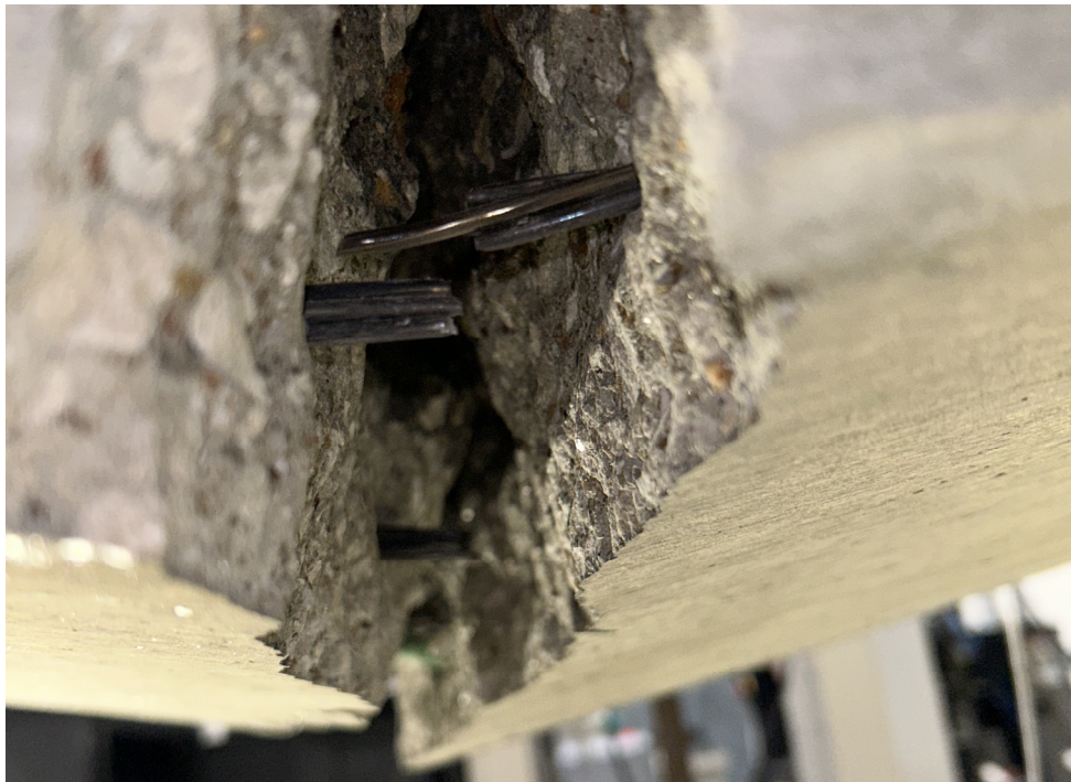
Figure 41: 8-foot 7-Wire Strand Failure
