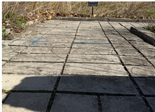
Fig. 4.21 Permeable pavers (Goold 2025)
