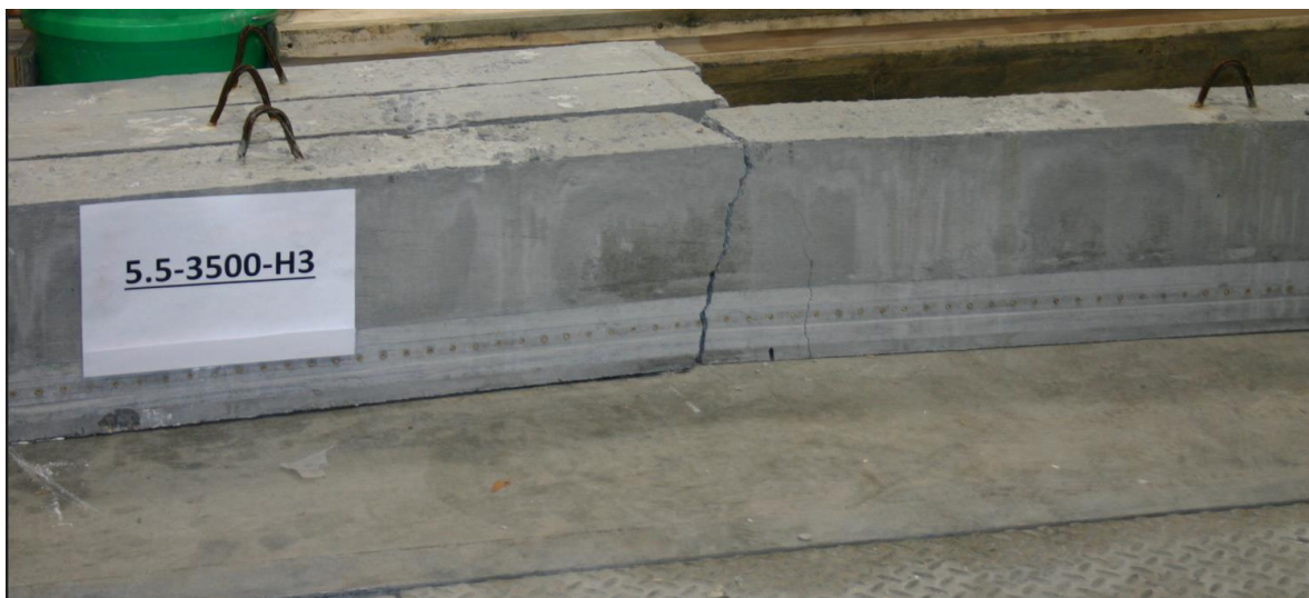
Figure D.6: Broken Beam Failing Through Strand Rupture.
