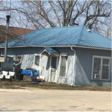
Figure 3.3.19 Dilapidated: A dwelling unit that suffers from excessive neglect, appears structurally unsound and not safe for human habitation, and may not be feasible to rehabilitate.
