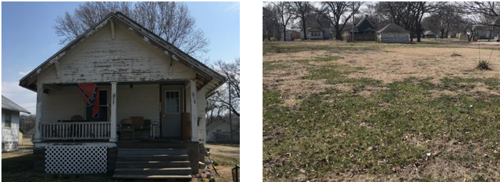
Figure 3.6.16 (Left & Right) Conditions Photos These photos display the current condition of two properties in the neighborhood. Photo on the right is vacant, and the left is dilapidated. (Marysville Housing Survey, 2019)
