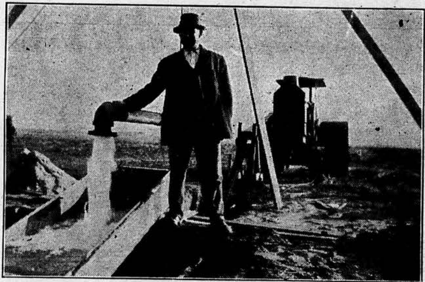
Running a Test on a New Plant; the Pumps Need to be Operated More on Kansas Farms than They Were Run This Year.
