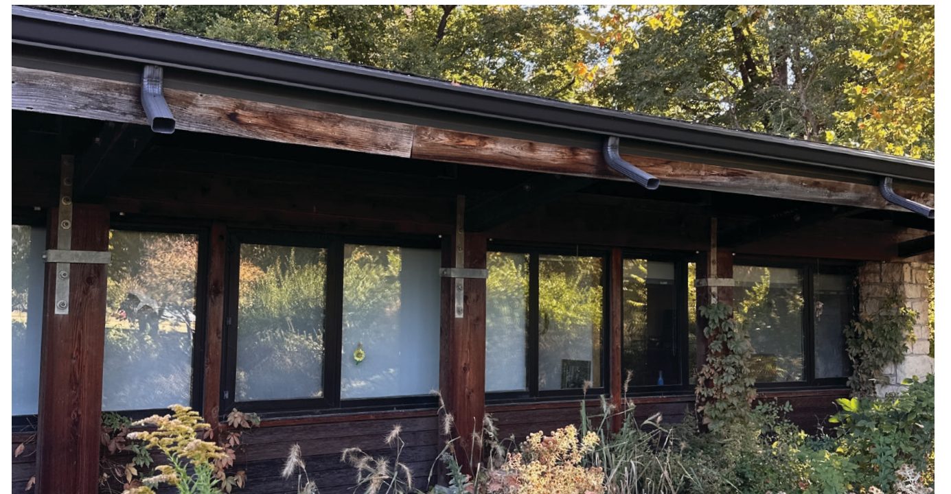
Figure 2.20 Rain-Bowls and Salvaged Limestone Splash-Pads are used to Dissipate Rooftop Runoff. (Tilley 2024).
