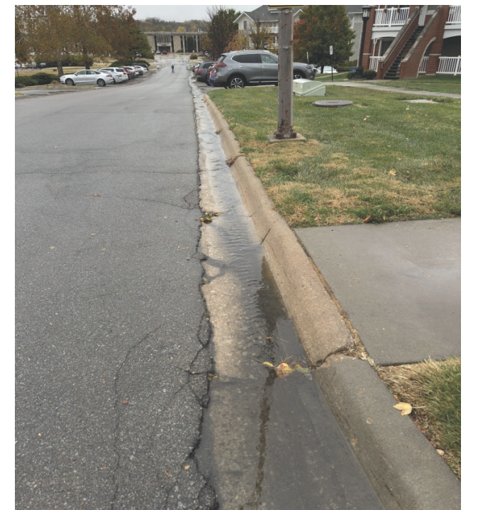
Figure 2.15 Rain Event Drainage along Kerr Drive (Freelove 2024).
