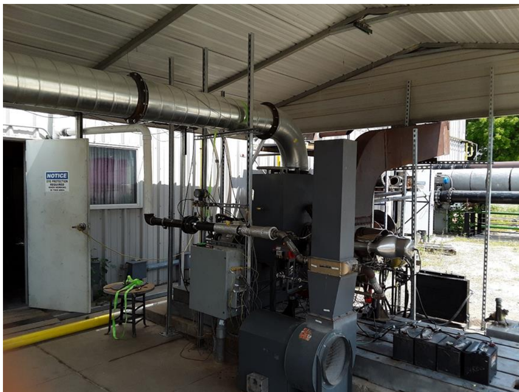
Figure 43-Allison 250 C28B engine test facility
