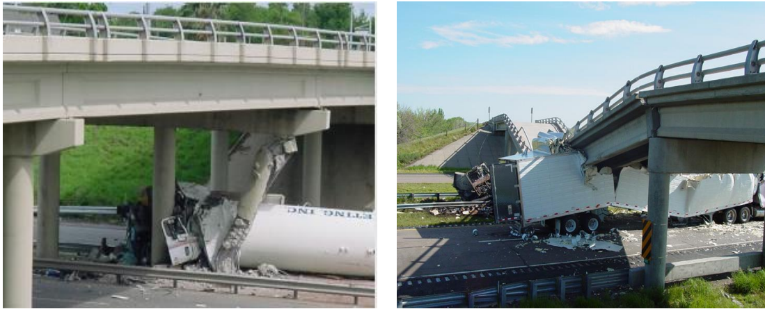
Figure 1-1. Failure of bridge structures due to vehicle collision events (N. Nemec, [3])
