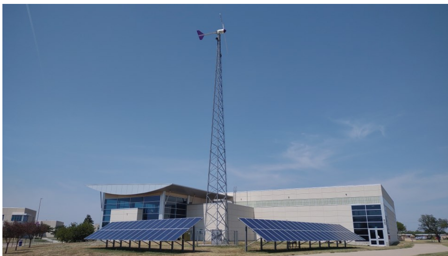
Figure 1.13. A picture of a renewable power system at K-State Salina consisting of 24 kW of PV panels and a 10-kW wind turbine
