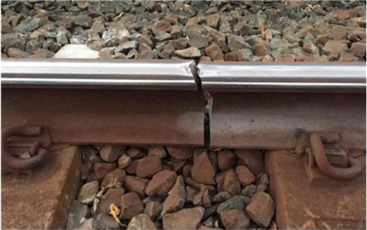
Figure 1.2 Fracture in Cold Weather 2
