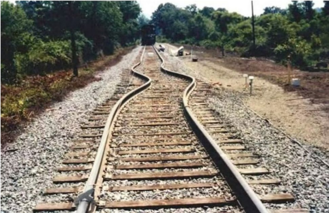
Figure 1.1 Buckling in Hot Weather 1
