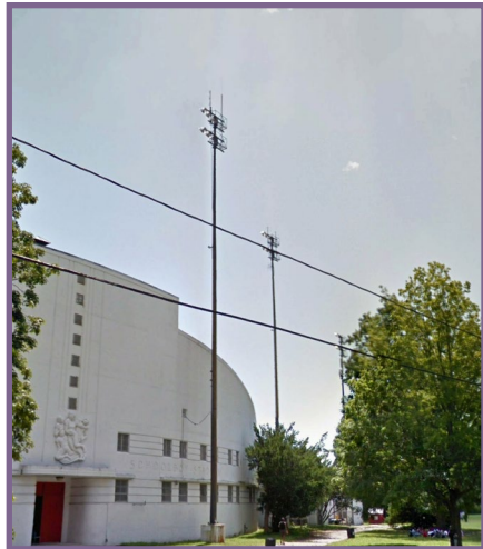
Figure 5.12.3: Existing Service Lighting | By Author
