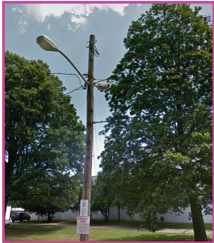
Figure 5.12.1: Existing Pedestrian Lighting | By Author
