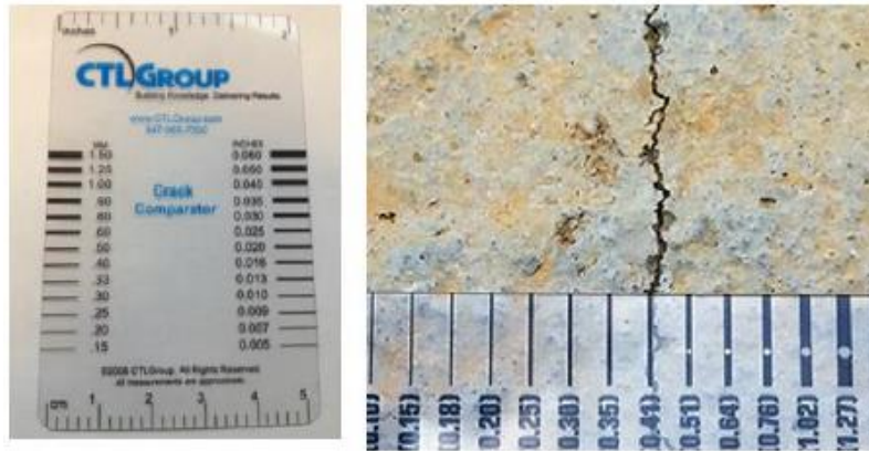
Figure 59. Crack measurement through crack comparator
