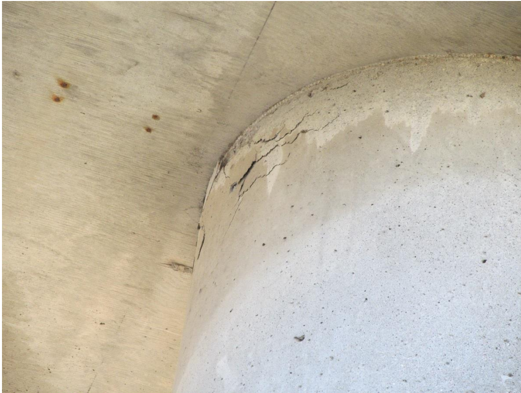
Figure 18: Concrete Distress at Top of Pier
