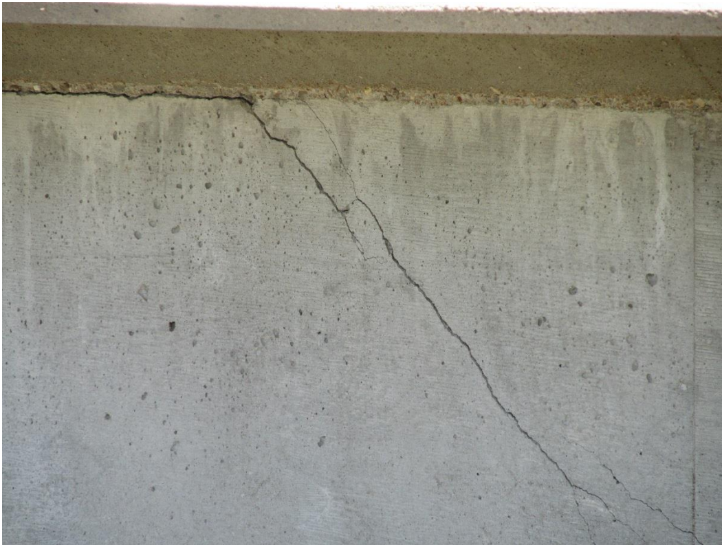
Figure 7: Shear Crack in Web of Box Girder
