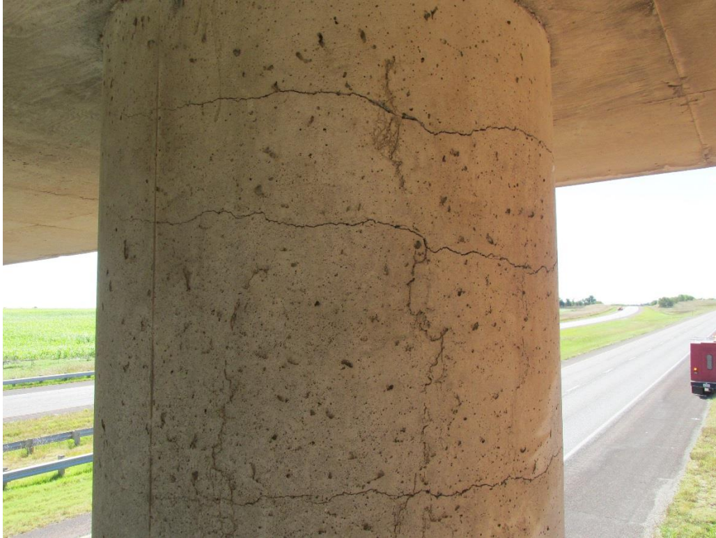
Figure 8: Radial Cracks at Top of Pier
