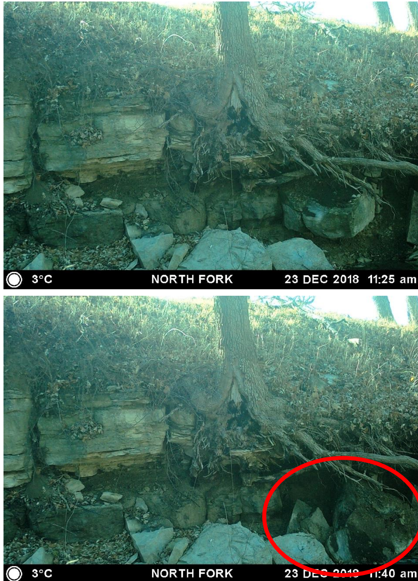
Figure A1 Example of mass block failure of limestone bedrock from the channel bank at the North Fork downstream site (red circle). The bottom image was captured 15 minutes after the top image.
