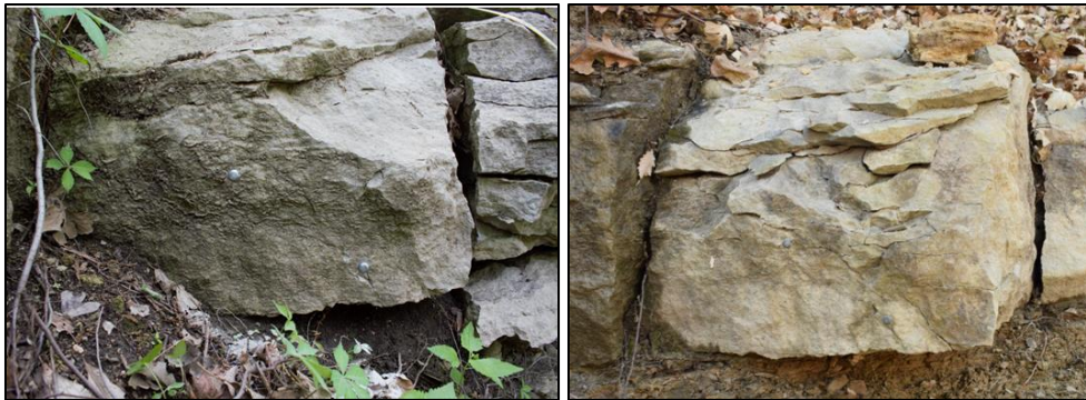
Figure 6.2 Limestone layer in the channel bank at the upstream North Fork site on May 16, 2018 (Left) and November 16, 2019 (right) with loosely held rock fragments, likely as the result of abrasion.
