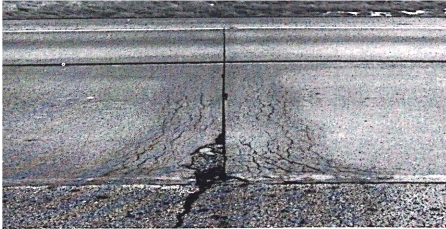
Figure 2-4 Development of D-cracking along joints (Schwartz 1987)
